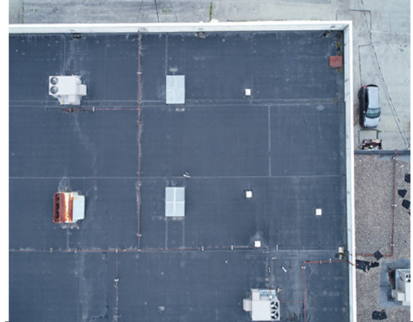
#18: SECTION B (B1,B2,B3,B4). VISABLE WATER LINES FROM ADJOINING PROPERTY HVAC UNITS.
