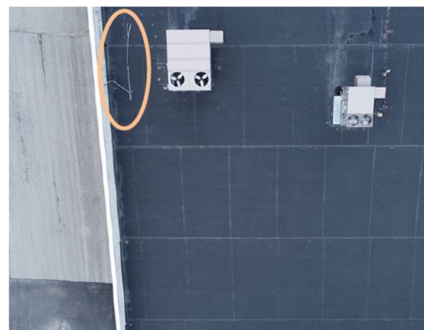
#20: SECTION C (C1 AND C2). VISABLE WATER LINES FROM BOTH HVAC UNITS. DEBRIS ALONG NORTH SIDE EDGE OF ROOF (ORANGE CIRCLE).
