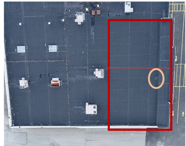
#22: SECTION F – SUSPECT DEBRIS ALONG WEST WALL (ORANGE CIRCLE).
