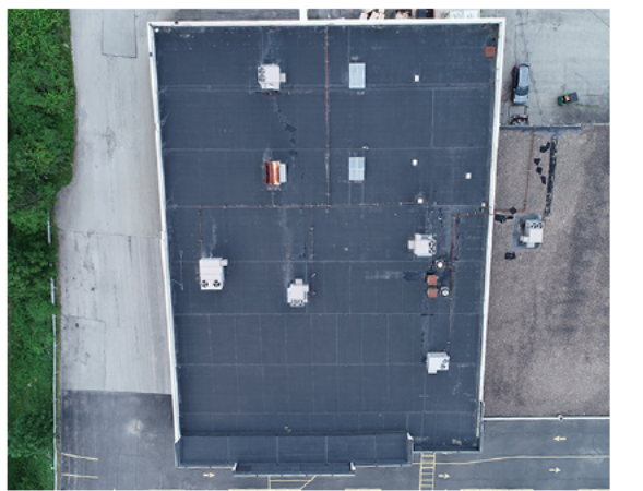
#12: BIRDS EYE VIEW OF STRUCTURE. VISABLE WATER LINES AROUND HVAC UNITS.
