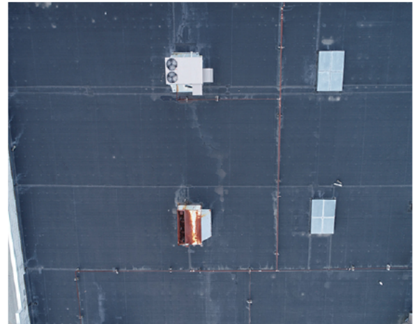
#14: SECTIONS A AND B (A1, A2, B1, B2). VISABLE WATER LINES AROUND HVAC UNITS.
