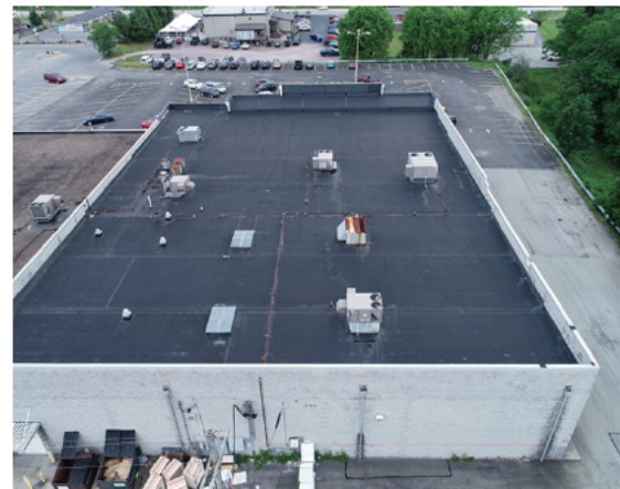
#8: EAST/BACK SIDE OF STRUCTURE SHOWING SECTIONS A,C,D,E,F. VISABLE WATER LINES AROUND HVAC UNITS.
